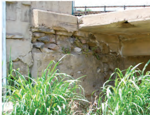
South abutment wall spall
