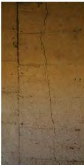
Typical pier vertical cracks
