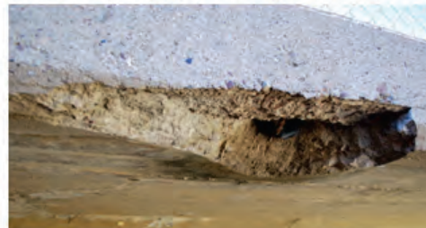
Sidewalk overhang spall, east edge, south end
