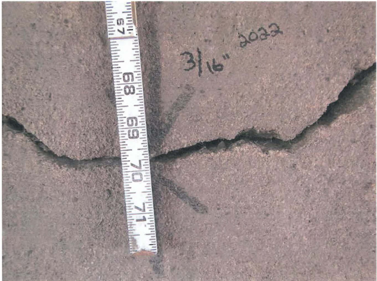
File Name : 09710-2022-05-06-Photo-10.JPG Description : Wide horizontal crack in Abutment 2
