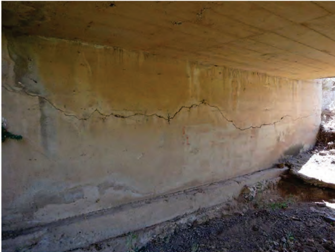
Photo No.: 5 File Name: 0971017e.jpg Descriptions: N abut. wide horizontal crack
